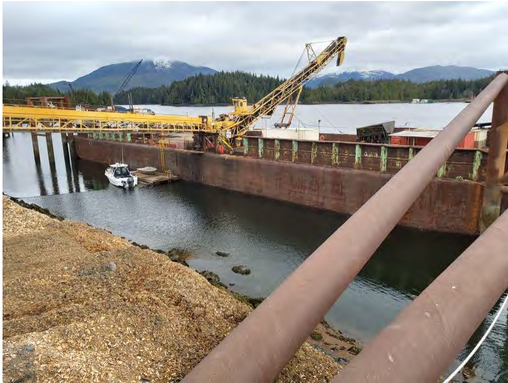
Figure 5. Photographs taken the foreshore near existing pile structure across from the south end of the barge.
