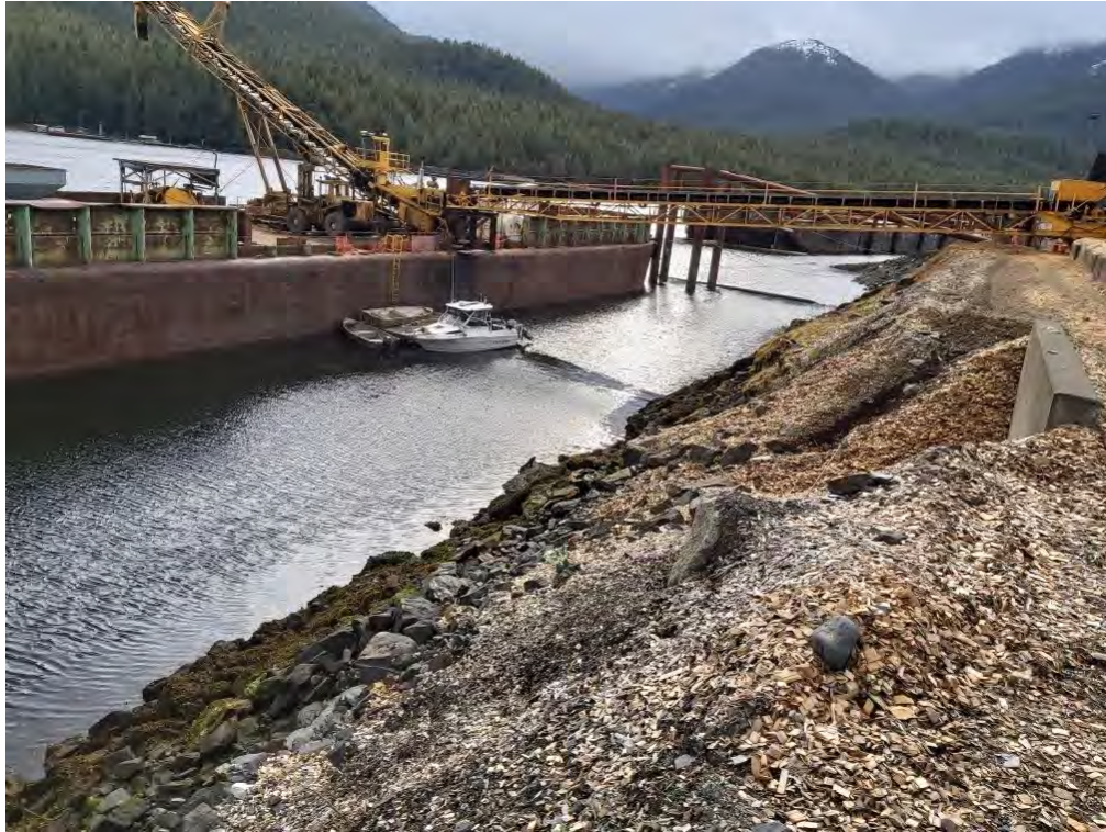
Figure 1. Photographs taken the foreshore near existing pile structure across from the south end of the barge.
