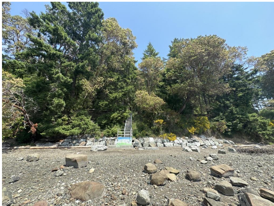
Photo 8. North view of riprap placement at CRD beach access near 431 Baker Road. May 30, 2023.
